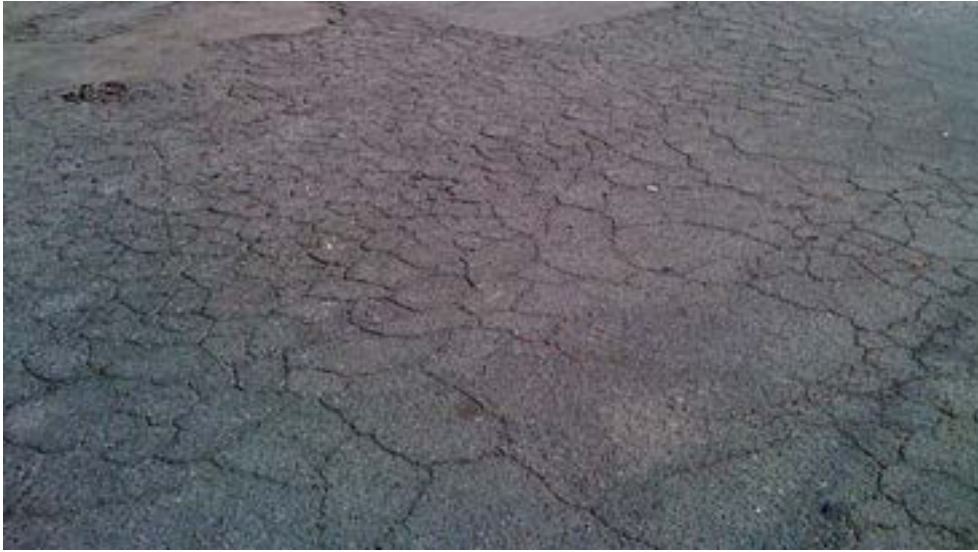
Fig. Alligator Cracking
