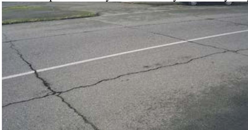
Fig. Joint Reflection Cracks
