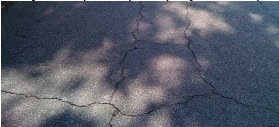
Fig. Block Cracking
