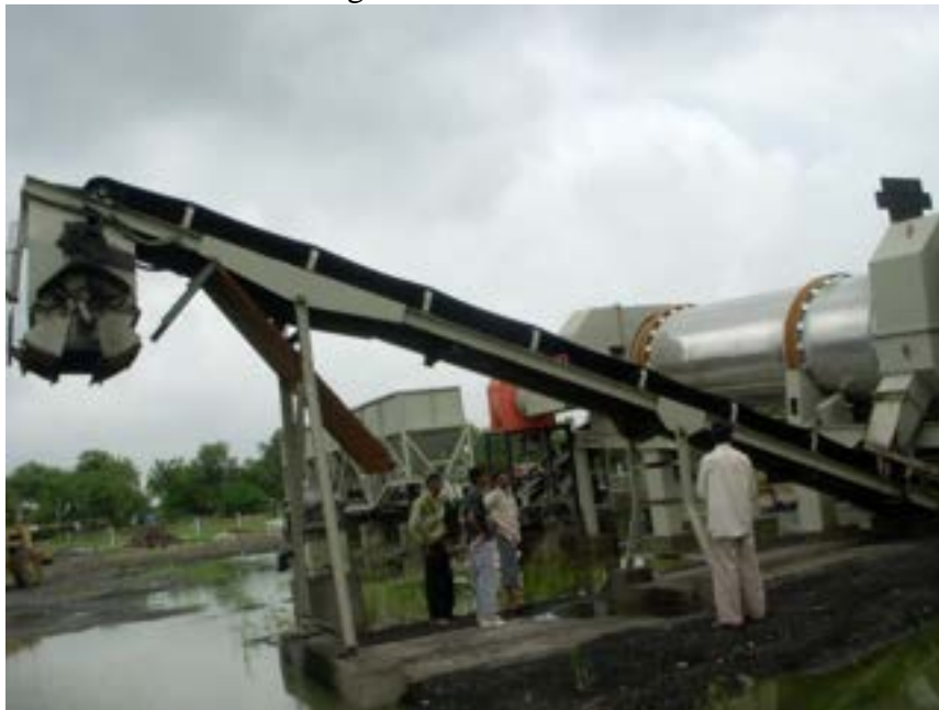
Fig. Load Out Conveyor
