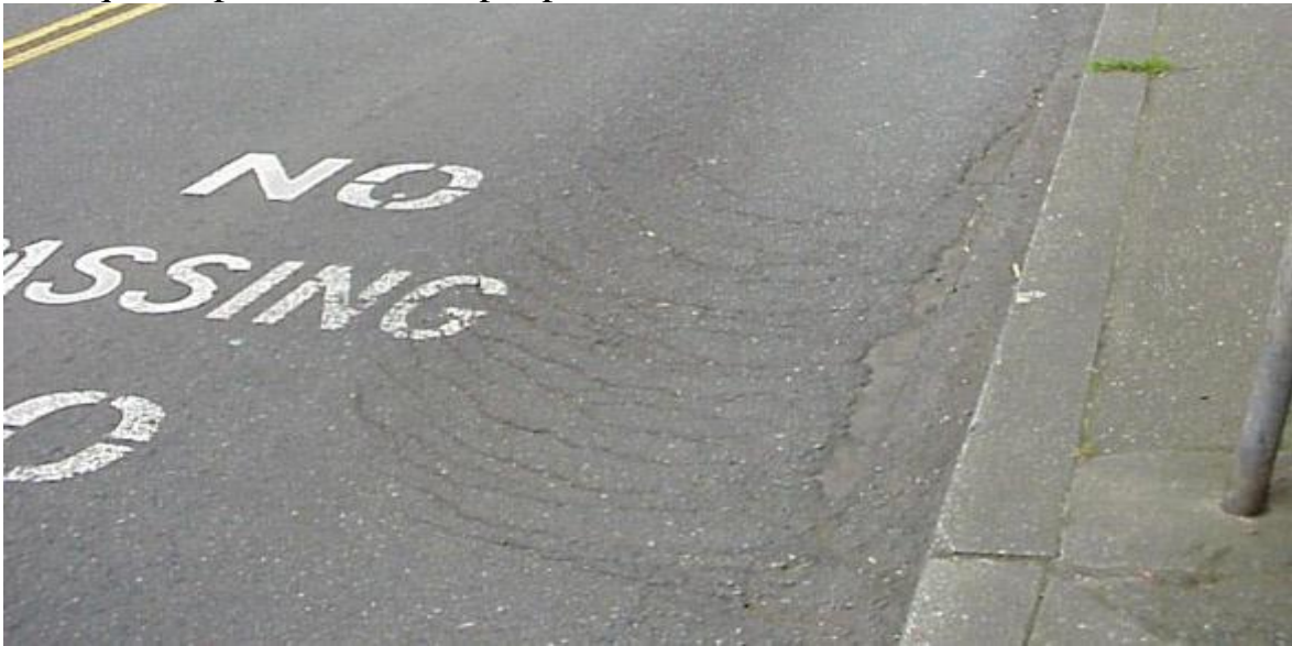
Fig. Slippage Cracks
