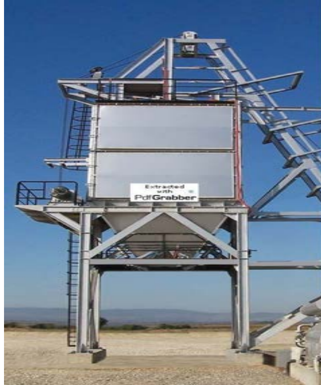
Fig.Hot mix storage silo
